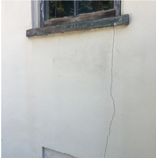
Typical Plaster Cracking
