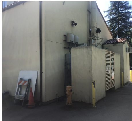
Cell tower equipment
