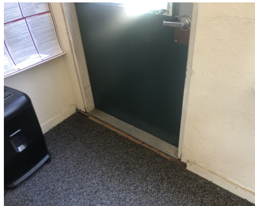
Water staining at threshold
