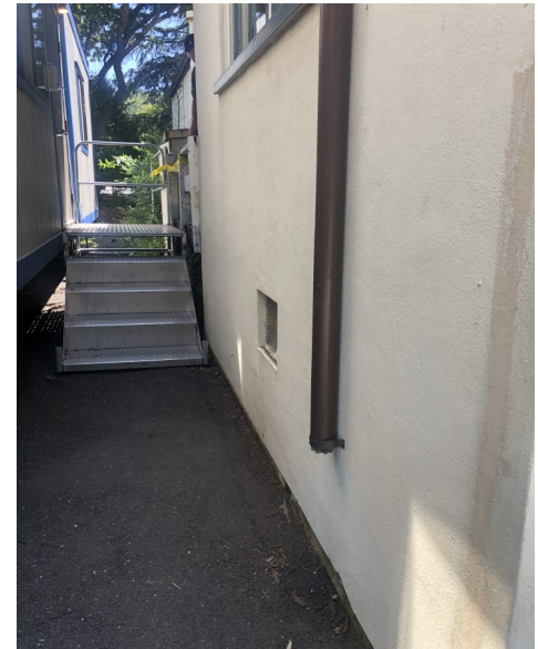
Unconnected rain water leader.
