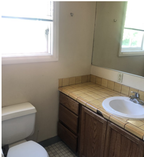
Broken counter top tile
