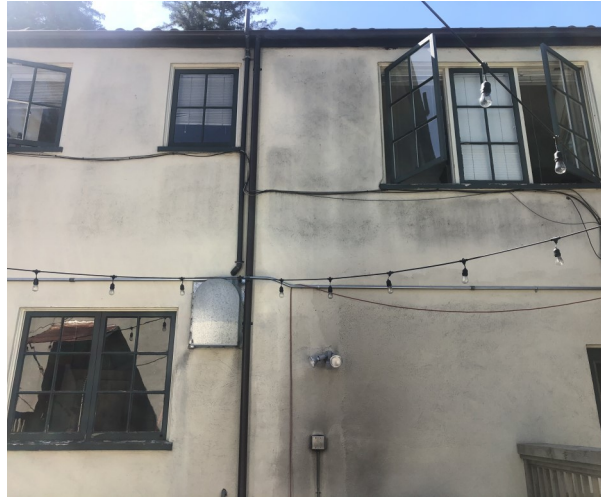
Exposed wiring, faded paint
