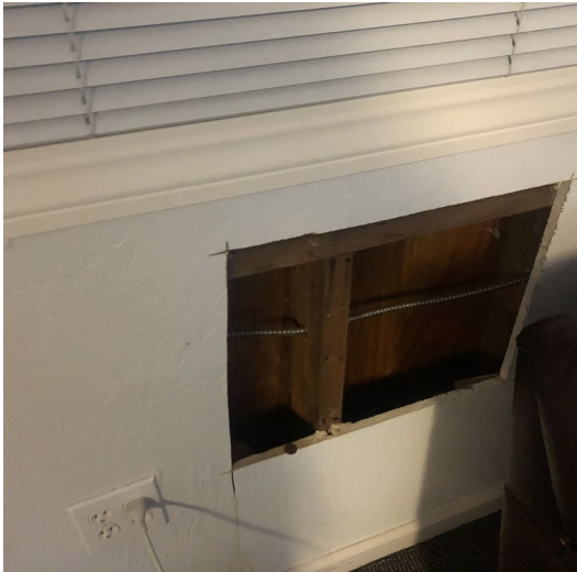
Portion of wallboard has been removed.
