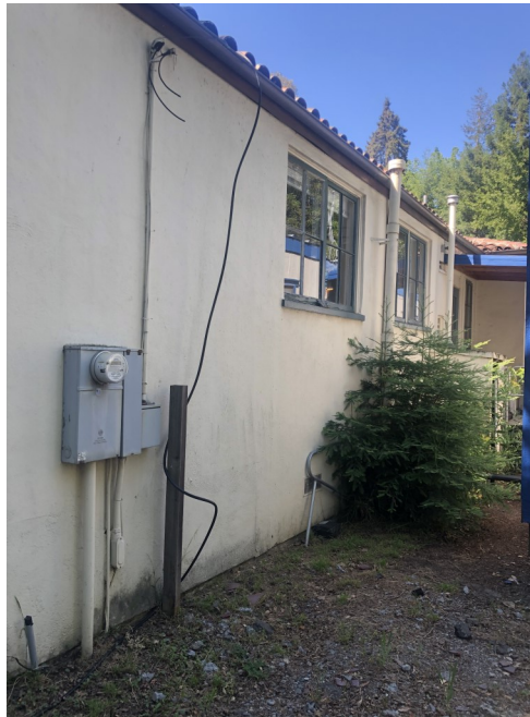
Soil contact with plaster
