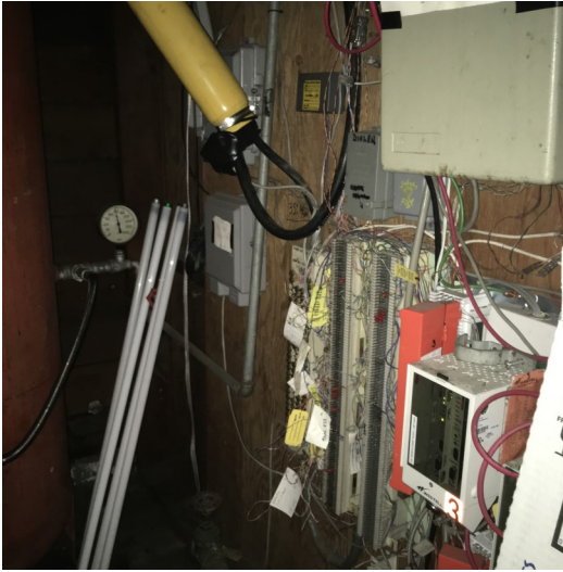
Exposed wires and unclear pathways
