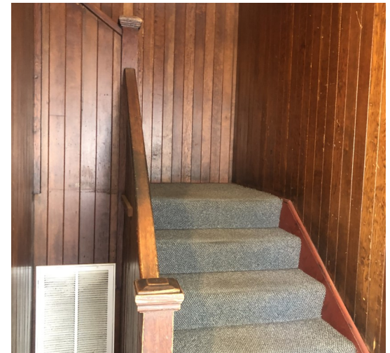
Non-compliant ADA stairs
