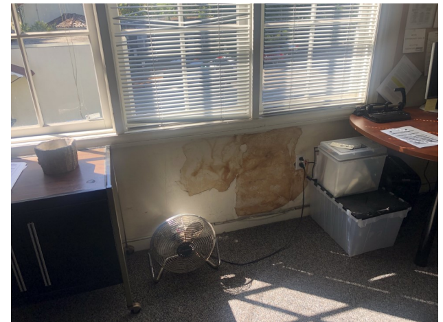
Water damage at exterior wall
