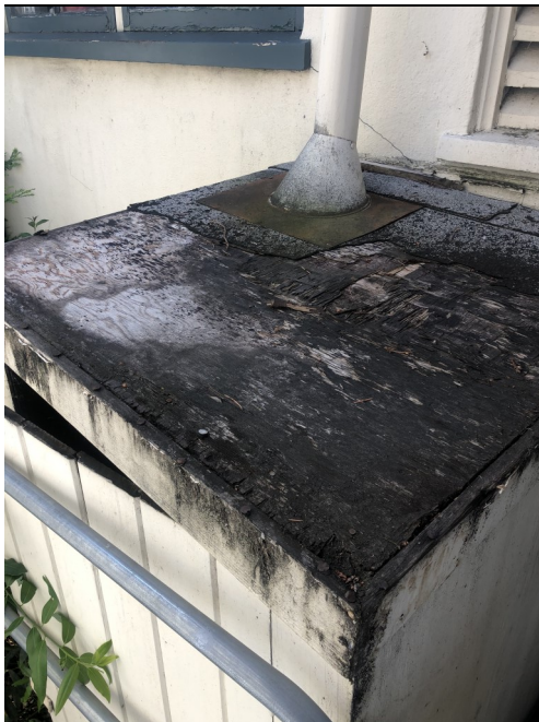
Roofing needs replacement
