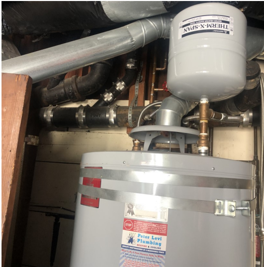
Fire House Water Heater
