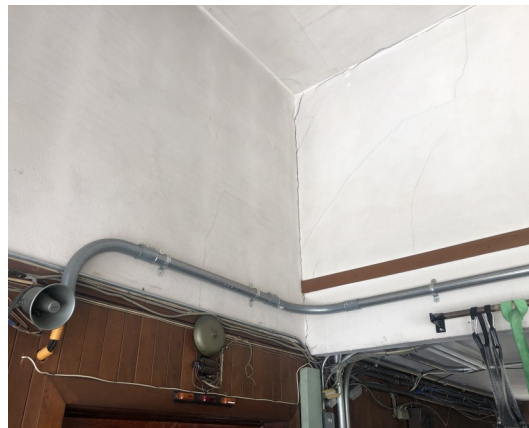
Interior plaster cracking
