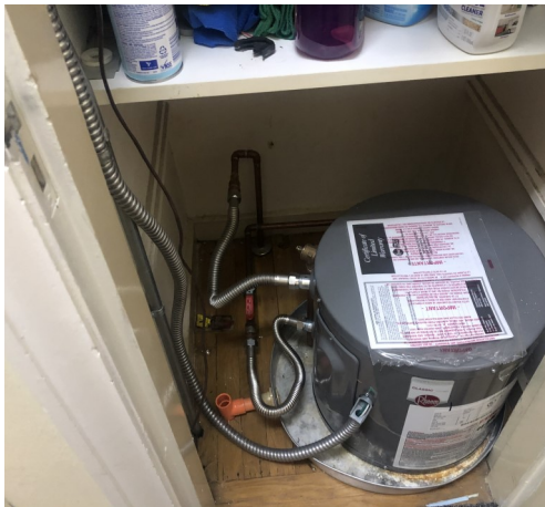
Police Station Water Heater
