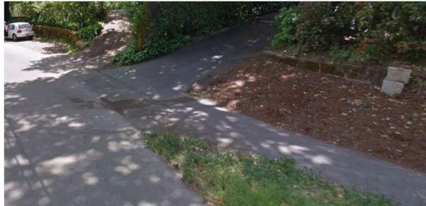
5 Eastbound sidewalk gap on Lagunitas Rd.
