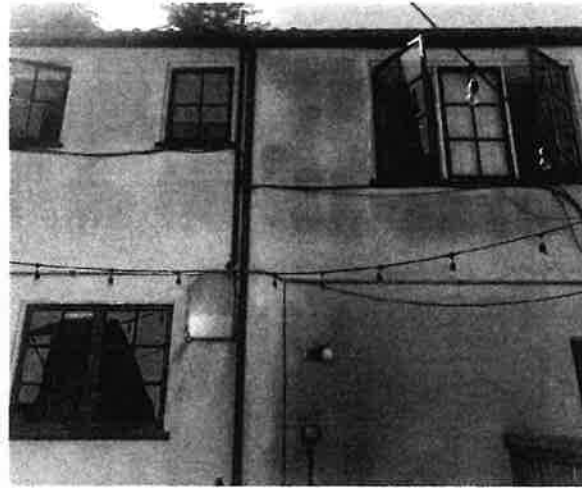
Exposed wiring, faded paint
