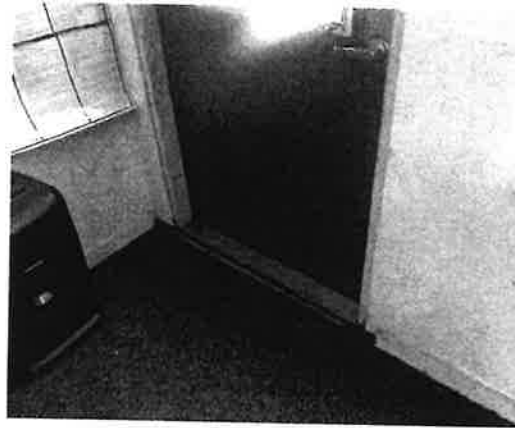
Water staining at threshold
