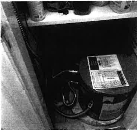
Police Station Water Heater
