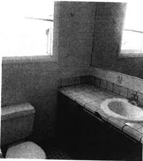
Broken counter top tile
