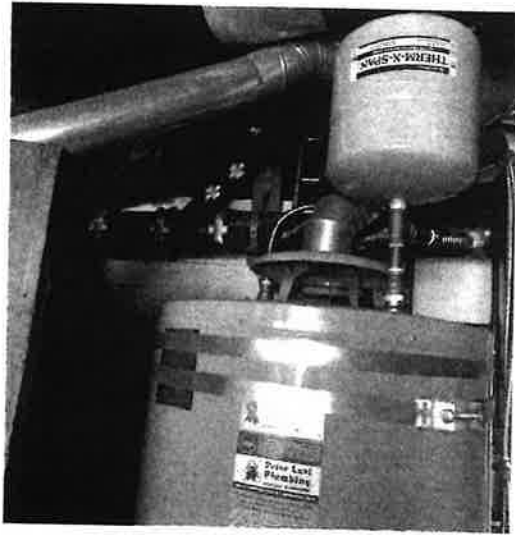
Fire House Water Heater
