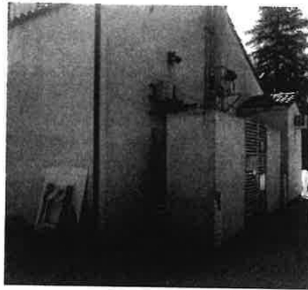
Cell tower equipment
