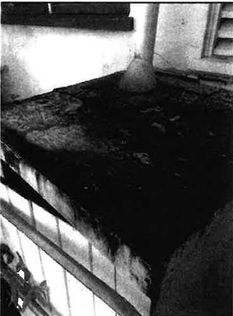
Roofing needs replacement
