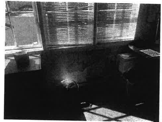
Water damage at exterior wall
