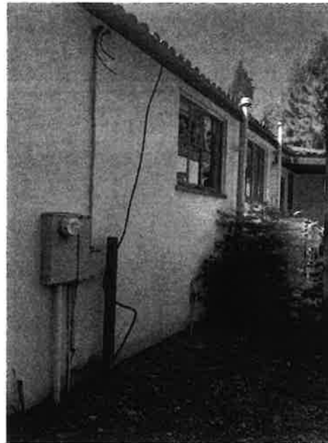
Soil contact with plaster
