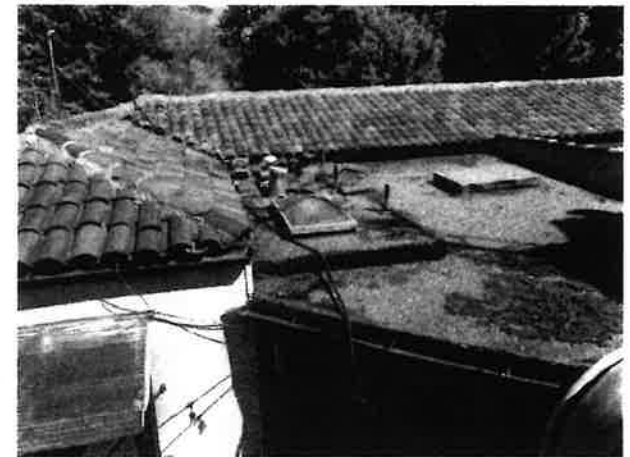
Roofing in need of repair, misc. exposed wiring.
